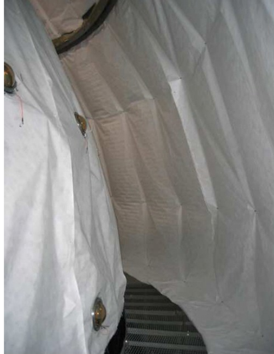
Fig. 5. The inner surface of the Water Tank covered with a layer of Tyvek. The Tyvek sheets improve light collection in the Outer Detector by reflecting the photons back into the water.
